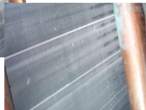
Below: Uncoated evaporator coil after 18 months; mildew on fins, patina on copper
